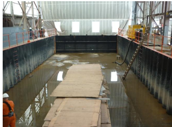
Dry dock gate in position
