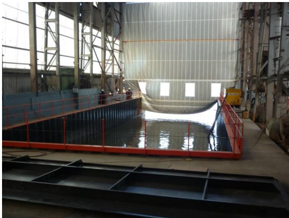
Dry dock fished with gate, shown in the foreground, ready to be lifted into
