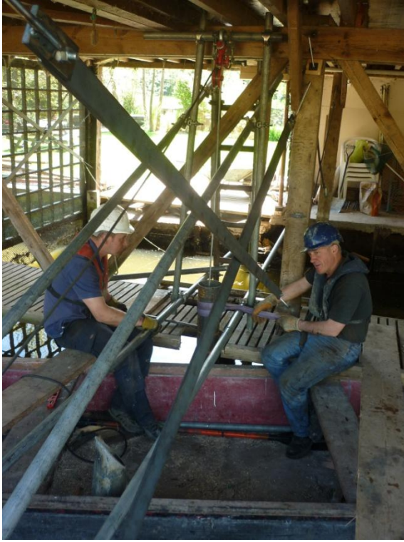
Using pulley blocks and bracing GTRP were able to install the bearing piles to a calculated set
