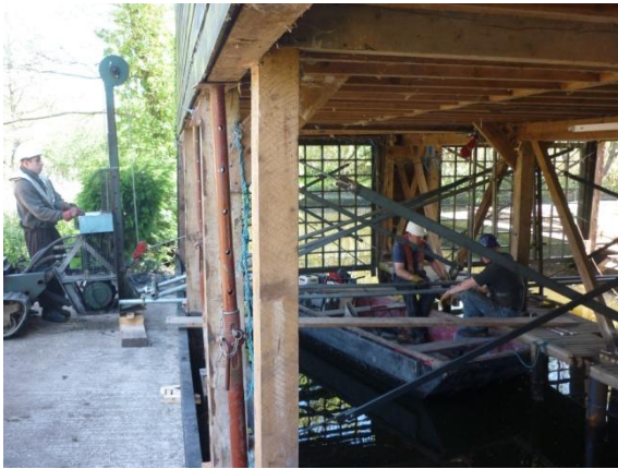
The mini piling rig standing outside of the building with the drop hammer wire running through pulley blocks
