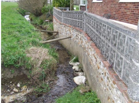
Flash flooding rose over the retaining wall and patio area causing the retaining wall to fail
