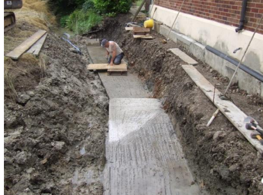
GTRP installed under-pinning to the bungalow to a depth below the adjacent stream bed level (note under-pinning evident in the picture). The stream was then diverted through pipe work but if flash flooding occurred the excess water is allowed to run through the concrete foundation works area
